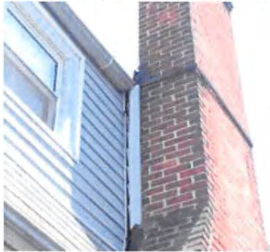
1.0 Evident chimney foundation structural failure / chimney pulling away from home
