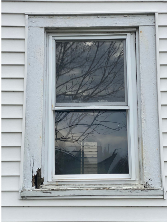
Existing windows in need of replacement
