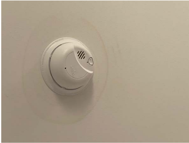
Water damage around smoke detector...this caused a short in the detector which set off all alarms on all three floors and the basement
