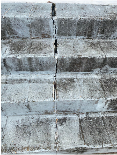
Porch Steps in need of repair
