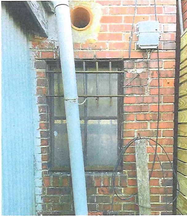
PHOTO "A" WINDOW TO BE REPLACED
