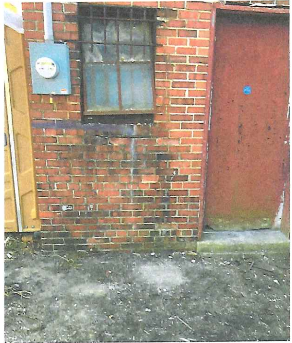
PHOTO "C" DOOR AND WINDOW TO BE REPLACED
