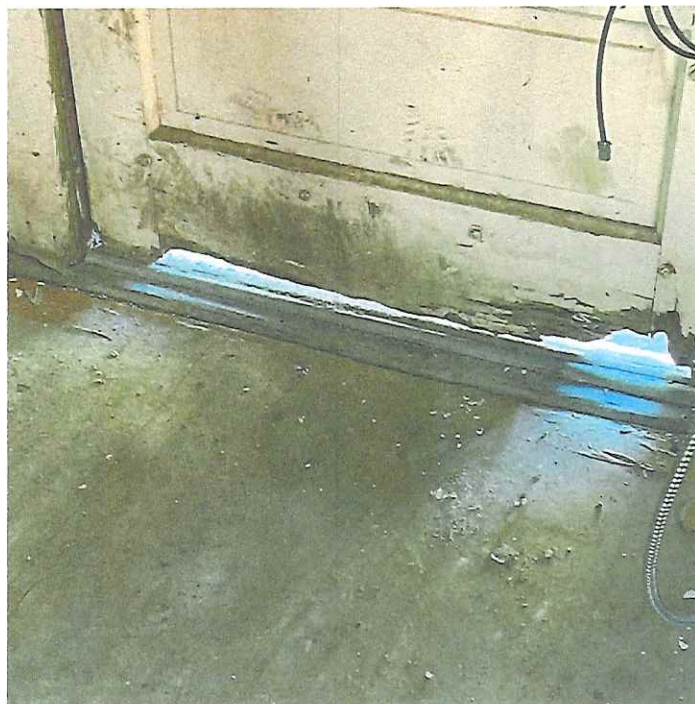
PHOTO "D" REAR DOOR FROM INTERIOR SHOWING ROT
