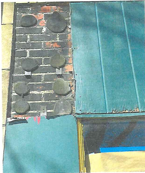
PHOTO "B" LEFT SIDE UNDER PLYWOOD
