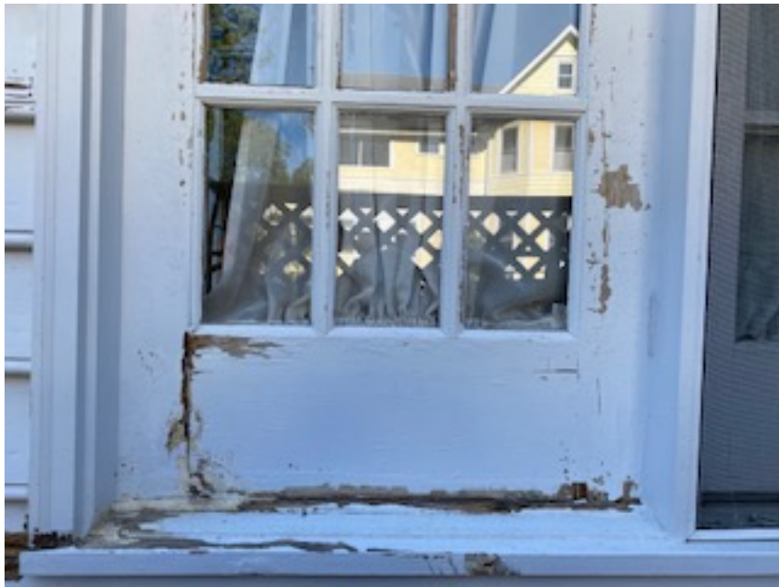
Figure 3 Rotting door -South side of building
