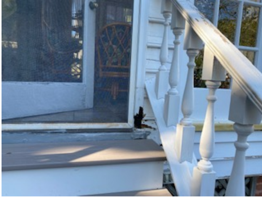
Figure 2 Rotting door frame - South side of building
