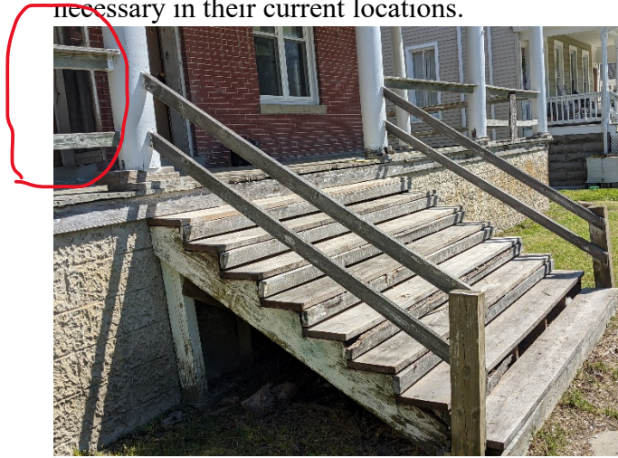
Figure 6-3A: Screens to a front door that will need repairing or replacement.
