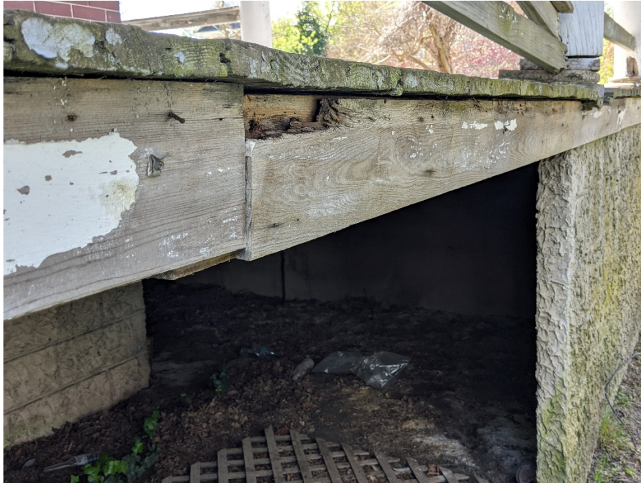
Figure 4-1A: Damaged and slanting banding boards and semi-rotten deck board sides.
