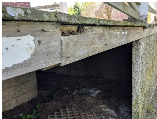
Figure 6-1B: Showing lattice on the ground, needing repair/re-installation.
