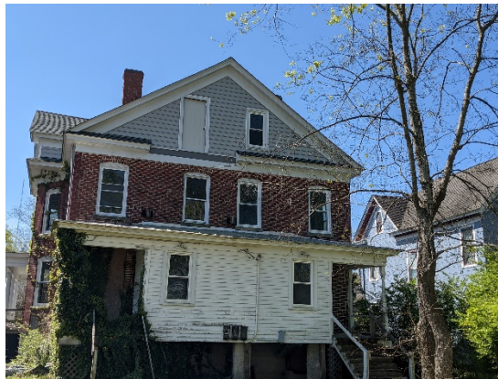
Figure 3-1B: Displaying door on 3 rd floor that must be replaced with a window – don't trip!
