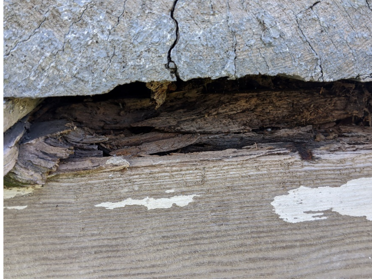
Figure 4-1B: Showing rot between boards and joists that needs repair with either wood or putty.
