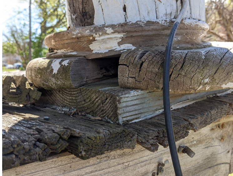
Figure 4-3A: Column Bases and exterior need touching up, repair, and replacement to the bottoms
