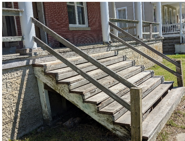
Figure 3-1A: Showing the railings needing touchup or replacement.
