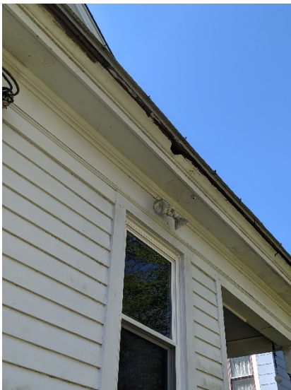
Figure 2-3B: Showing general wear and damage to soffit and fascia board that will need to be repaired.
