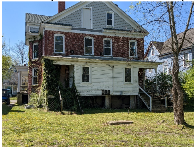
Figure 4-2A: Showing the stairs on the back of home needing extensive repair and restoration.
