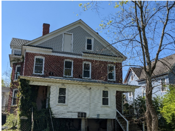
Figure 3-2B: Outside view of the rear of the residences to display the exterior windows condition.
