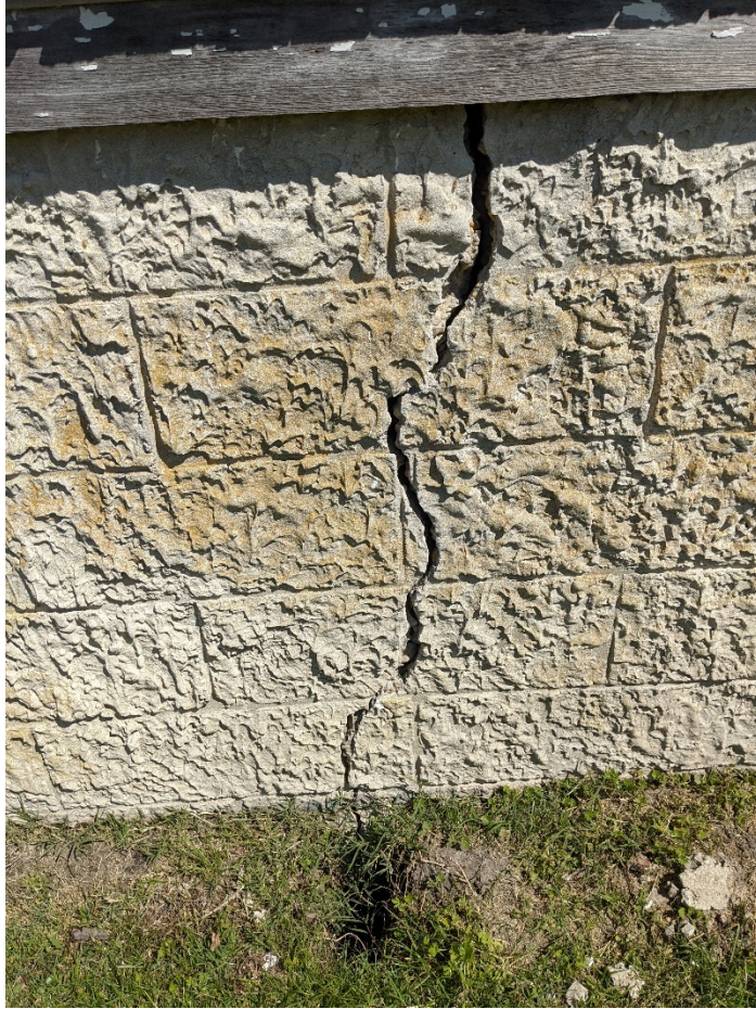
Figure 5-1A: One larger crack on the front of the home that must be repaired to match.
