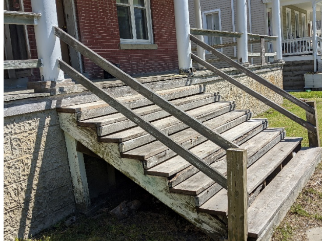
Figure 4-2B: Showing the front stairs that will need touchup and potential replacements of boards.
