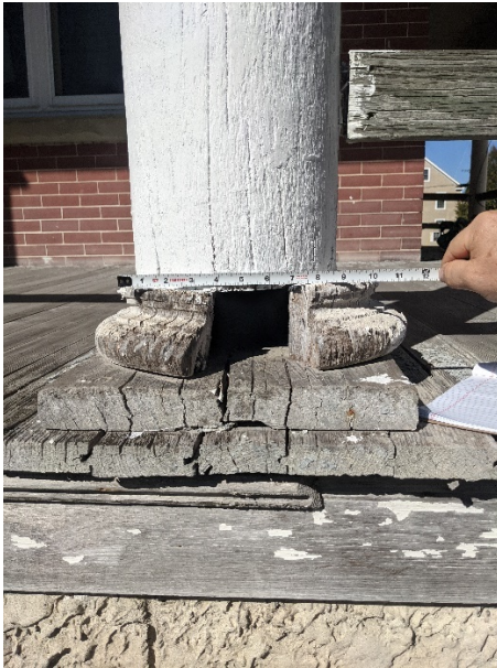
Figure 6a: Bases of the columns are near missing and in bad condition.
