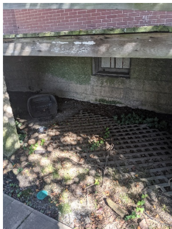
Figure 8: Showing Lattice that must be reinstalled and repainted.
