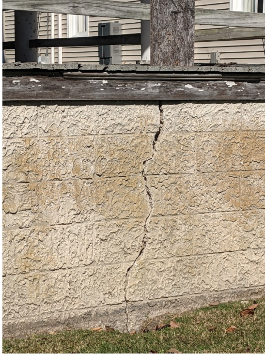
Figure 7: Showing Cracks in the Masonry that require point-up.
