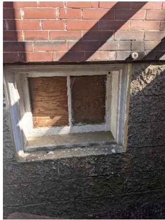
Figure 3a: Showing the basement windows boarded up and broken, needing restoration.
