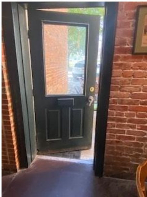
Opens out for access. Need protection from the elements
