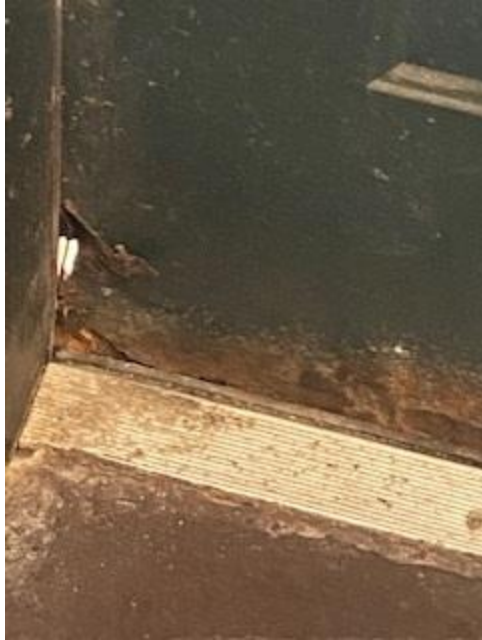
Totally rotted out. This is a standard metal door
