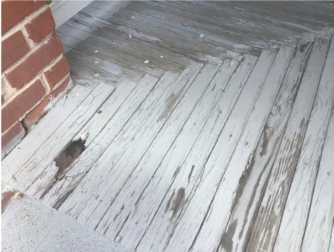
Photos of current porch condition
