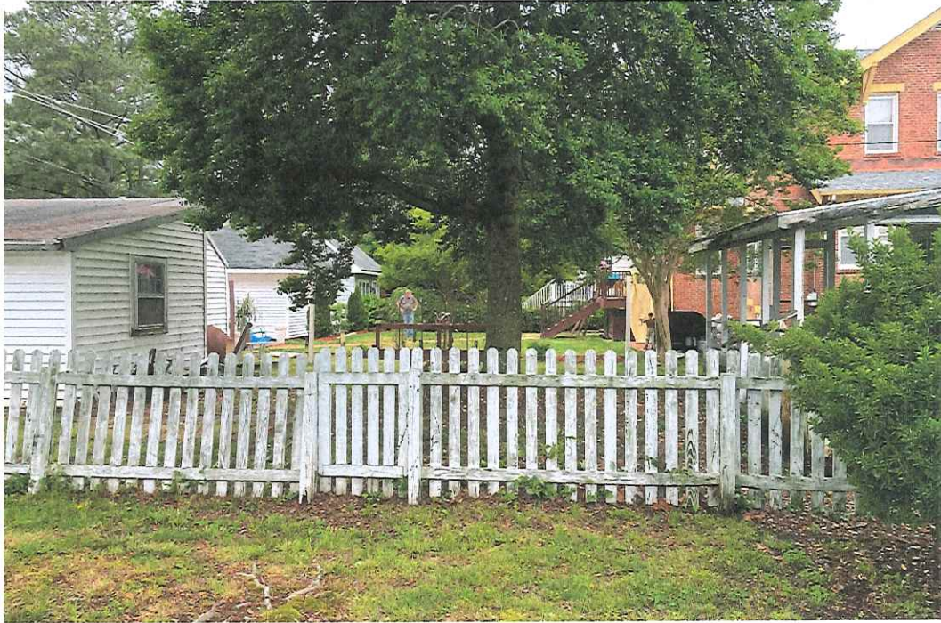
Existing Fence to be repaired and replicated
