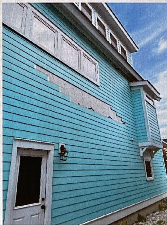
Missing Siding & Door #2
