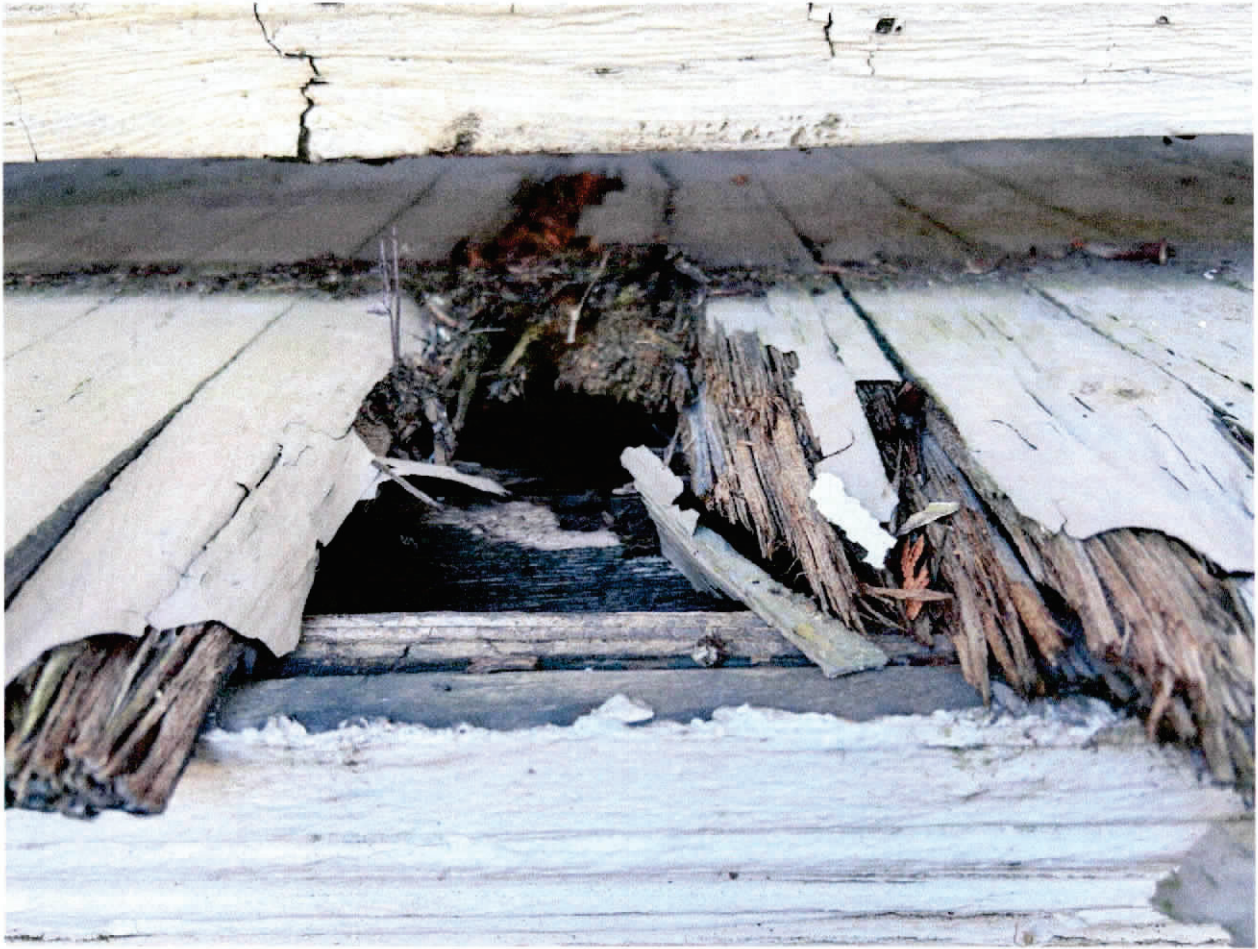
Front porch deck rot
