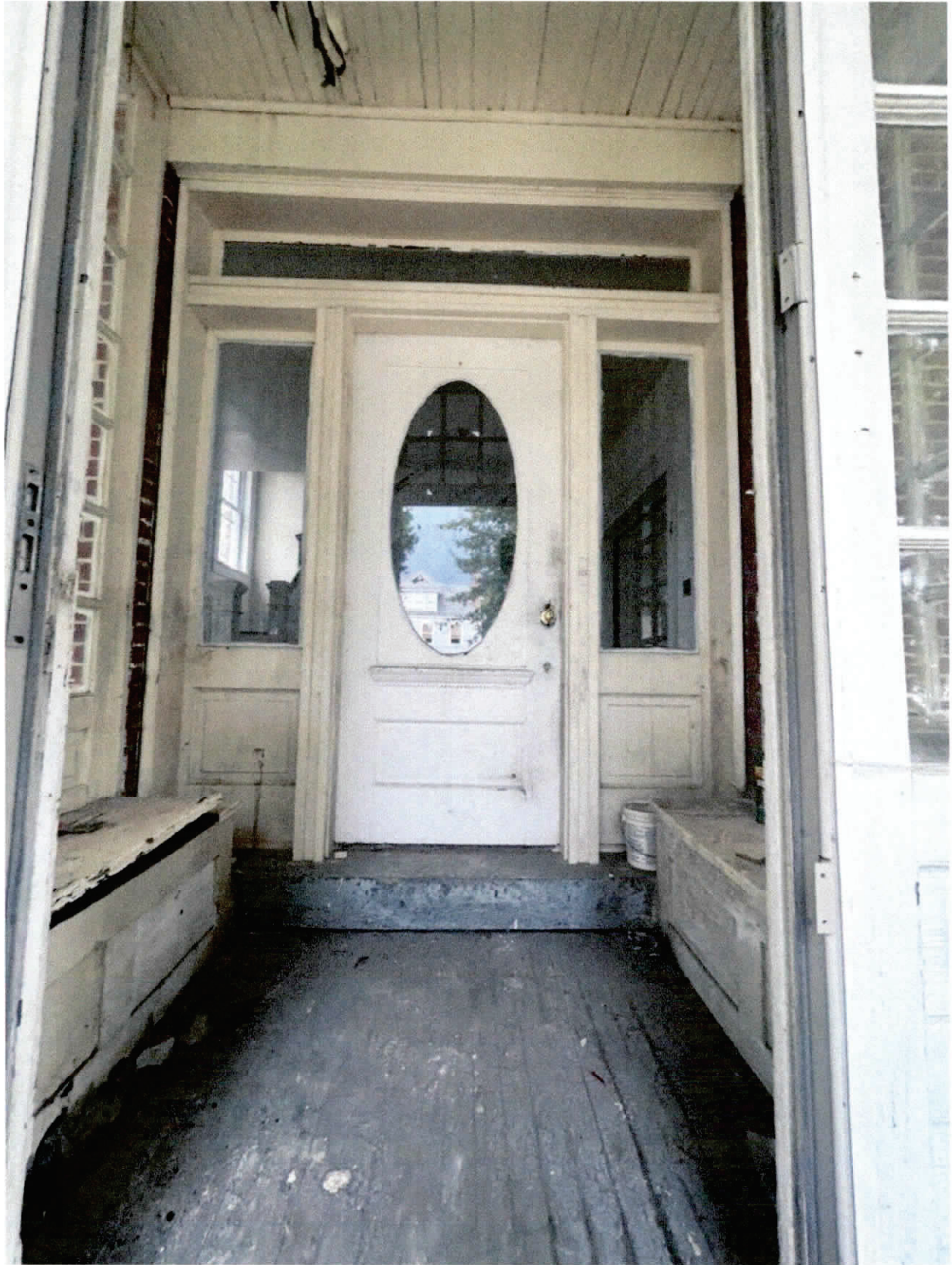
Front Porch Rot
