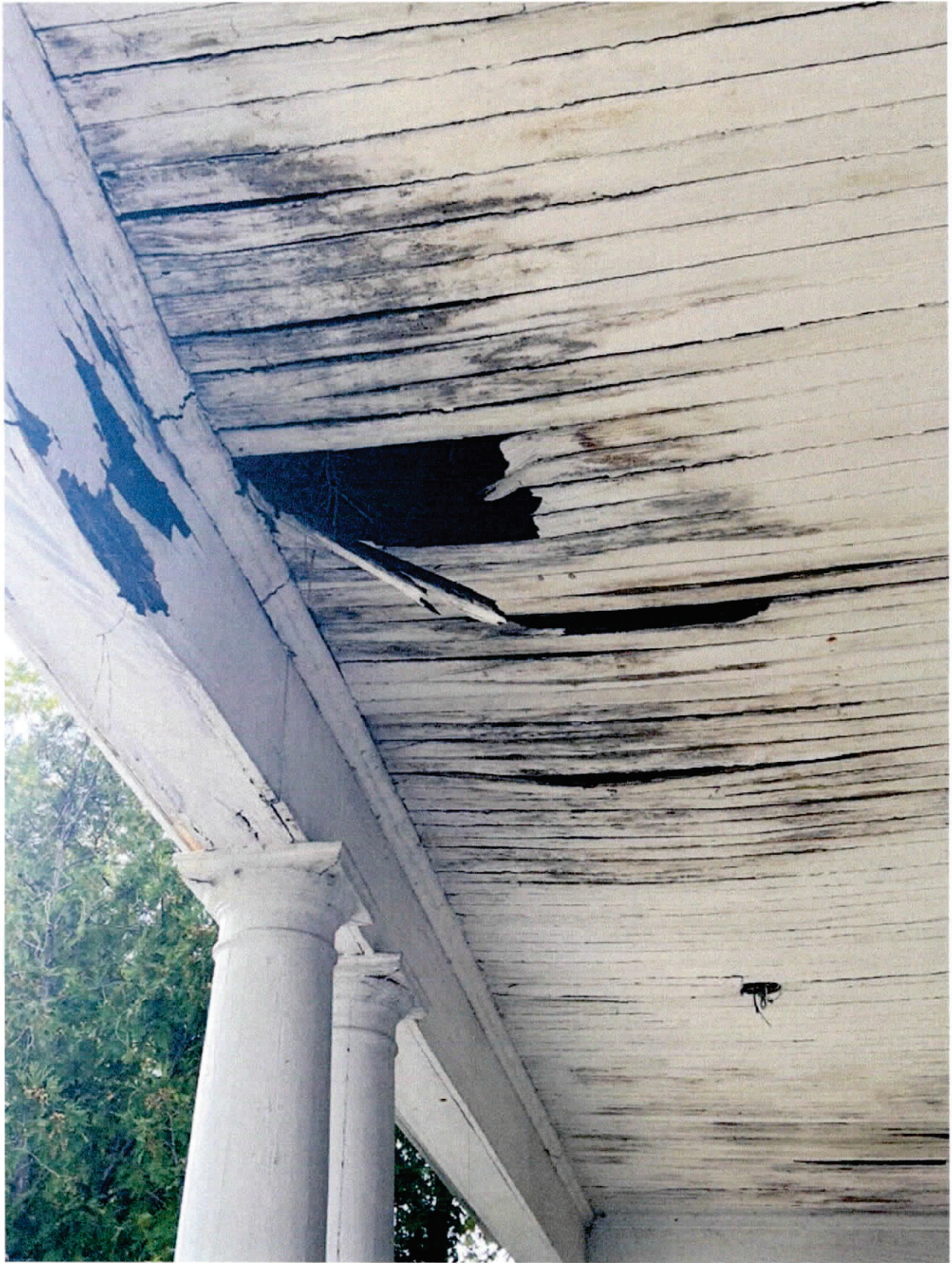
Front Porch Rot
