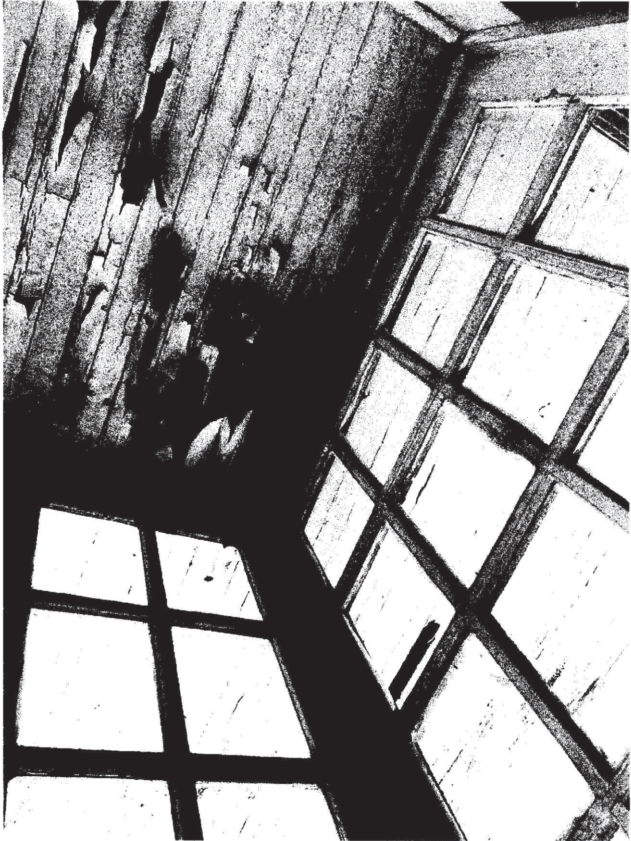
Front Porch Rot
