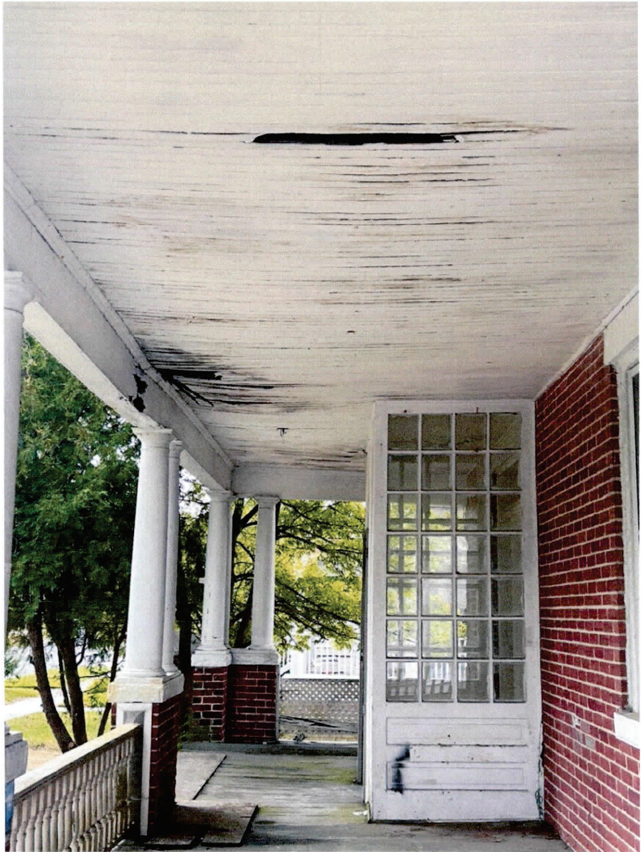
Front Porch Rot
