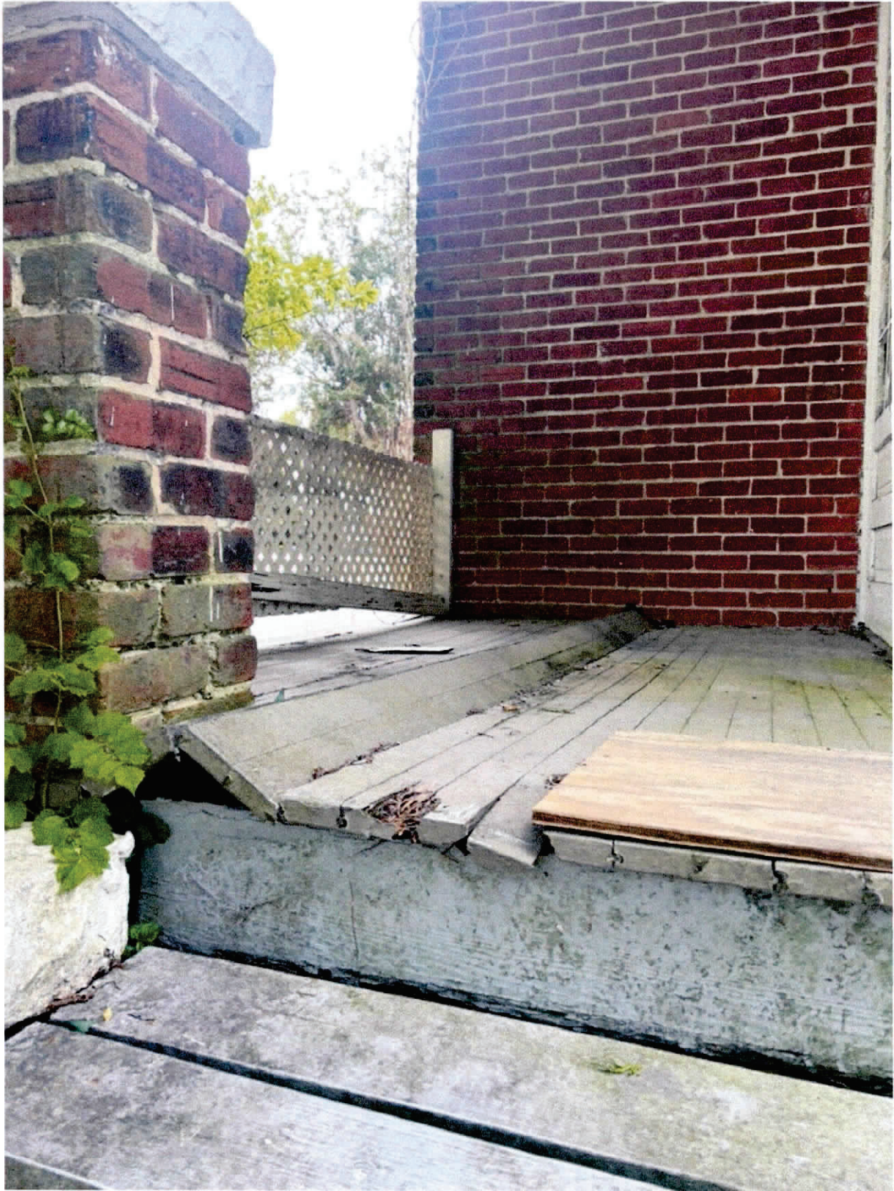
Front Porch Decking Rot / Disrepair
