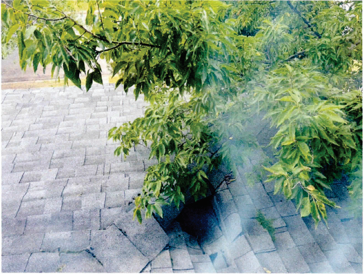
Hole in Porch Roof
