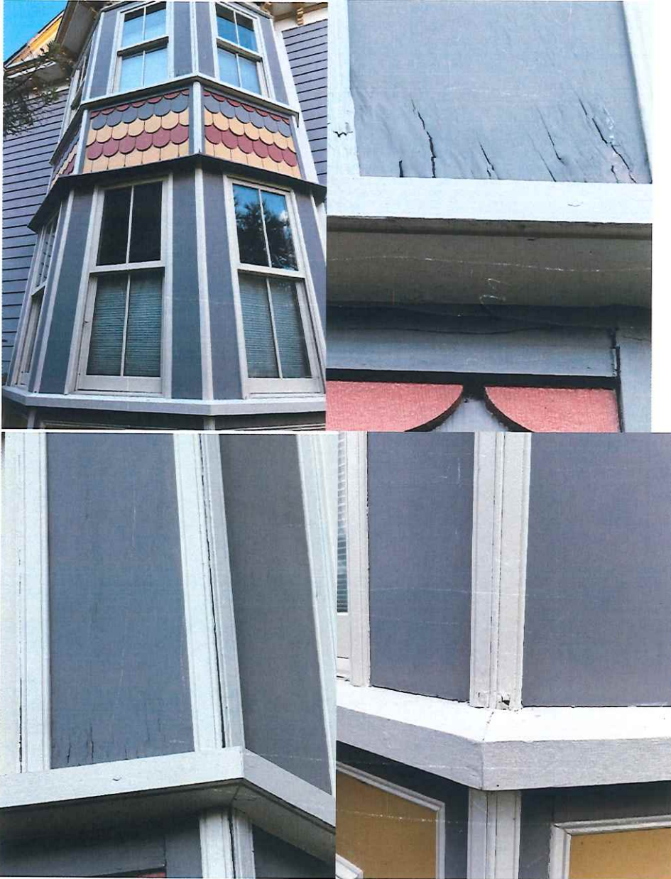
526 Tazewell Avenue Pictures of Wood Damage to Bay Window
