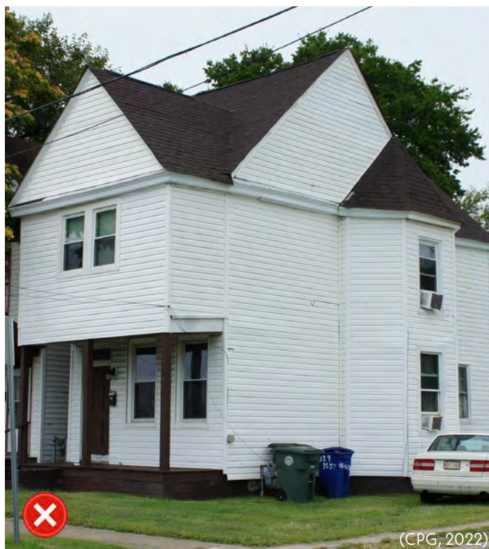
Figure 5.32 - The number of windows has been greatly reduced and altered on the primary elevation and exposed side elevation. This is inappropriate for the Cape Charles Historic District Overlay. (CPG, 2022)
