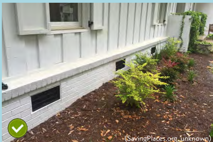
Figure 8.6 - Flood vents that allow water to move under the building is an example of wetproofing.
