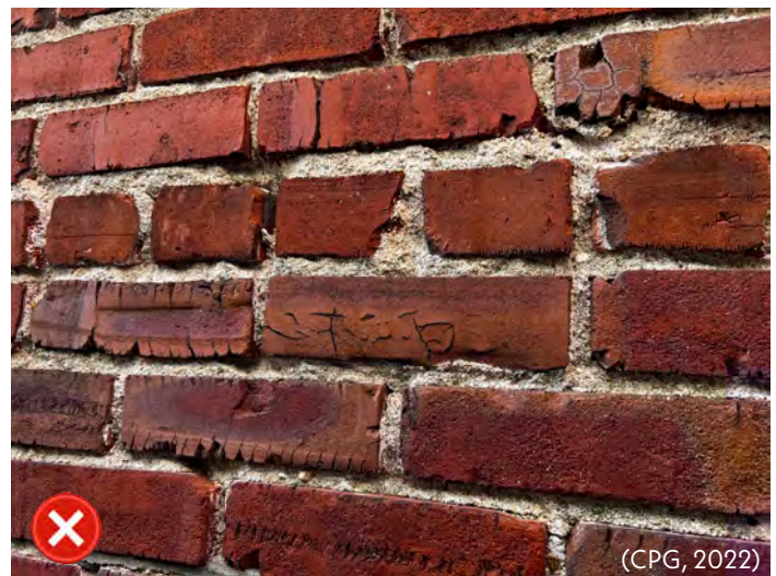
Figure 5.7 - Portland cement mortar has been applied to this historic brick wall. The hardness of the cement has caused the softer brick to compress and begin to crack and spall.
