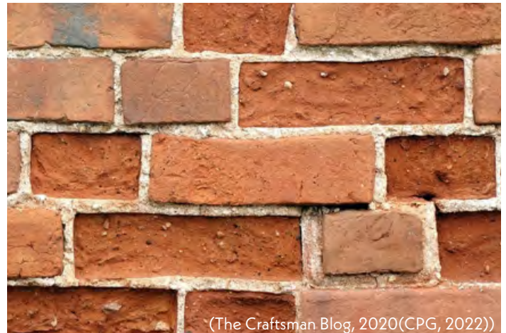
Figure 4.7 - Brick has surface layer, the brick face, that protects the softer, inside portion of the brick. When the brick face is damaged, which can occur when pressure washing at a high psi, spalling (shown above) occurs. The result is compromised bricks that flake and break away. When masonry requires cleaning, use a pressure of no more than 300 psi.
