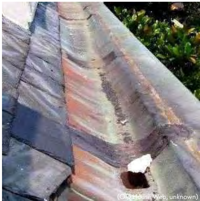
Figure 5.5 - An example of a built-in gutter in need of repair.
