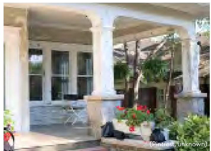
Figure 4.12 - While in need of minor repairs and new paint, this porch is in salvageable condition.
