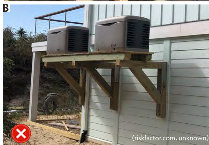
Figures 8.10 A & B - Exterior mechanical equipment needing to be raised should be located out of view from the public right-of-way and freestanding (A). Attaching brackets to a historic building (B) is not recommended as it can strain and damage the structure.
