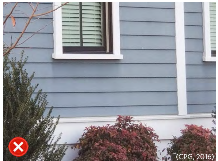
Figure 5.38 - The photograph above is of Hardie Plank material on a house. After 2 years, it has faded noticeably where the original color can be seen under the sill.
