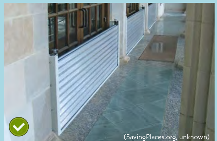
Figure 8.5 - Flood gates at the building's openings are an example of dryproofing.
