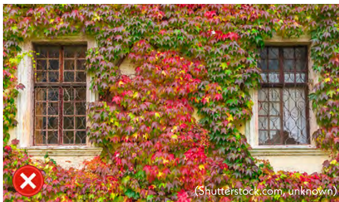
Figure 9.13 - Plants attached to historic materials can be detrimental to them. They hide possible deterioration and damage, impede repairs, trap moisture in their root system, and can weave into cracks making it difficult to remove. Using a trellis, frame, or wires installed near the building allows for the look, without the threat.
