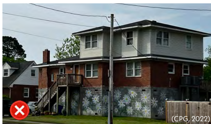
Figure 8.12 - Concrete block is exposed and a new modern stair/deck is disproportionate to the rest of the building. This is a dramatic and visually intrusive solution.
