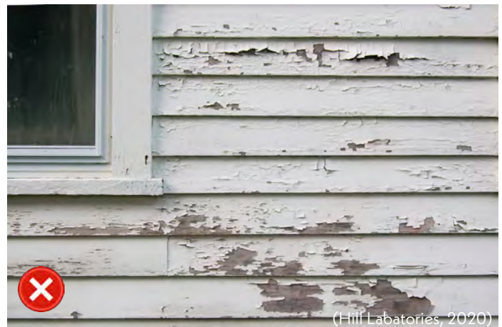
Figure 4.10 - This siding has weathered and peeling paint. It should be sanded down and repainted as soon as its deteriorating condition is noted so that the wood is not exposed to the elements.
