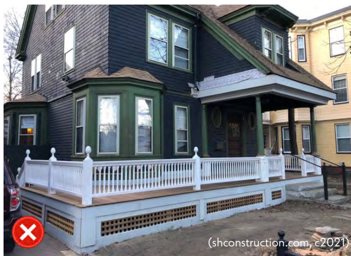
Figure 9.8 - Decks should not be constructed at the front of the building or attached to front porches, as shown above. It detracts from the historical features and creates a false sense of what the house historically looked like.
