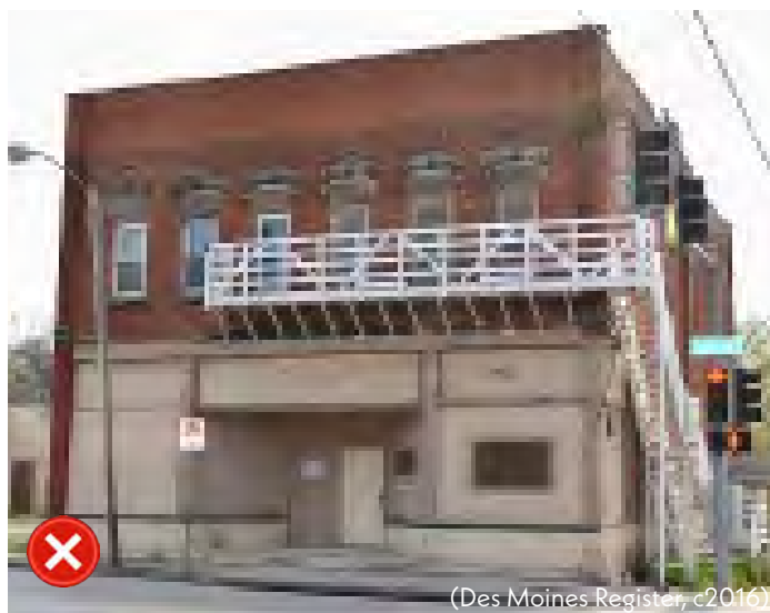
Figure 5.28 - This is an example of an inappropriate storefront modification. The display windows have been covered with modern siding, and the exterior stairs and balcony are an inappropriate alteration.
