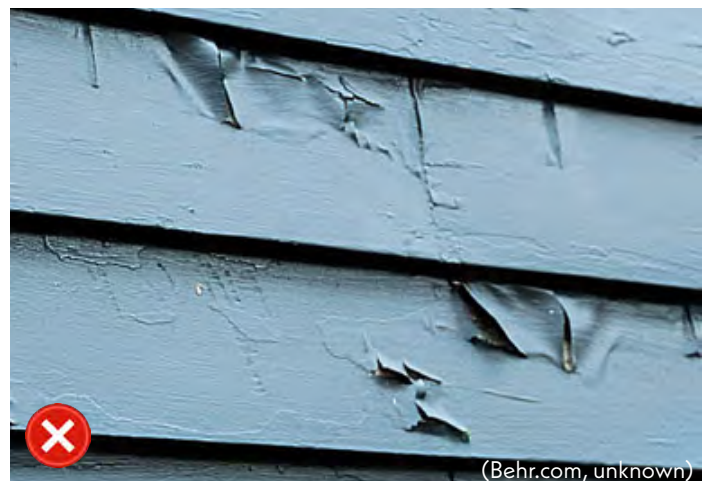
Figure 4.11 - The siding above has been painted when the wood was either too wet or there was a high level of humidity, resulting in bubbles and peeling of new paint.
