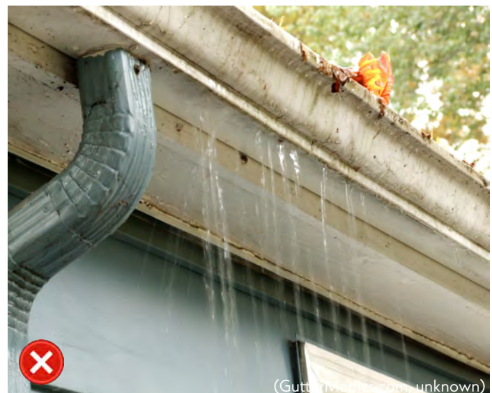
Figure 4.1 - The gutter shown above is clogged with leaves. These types of issues are easily fixed and will avoid excess water infiltration at the foundation.
