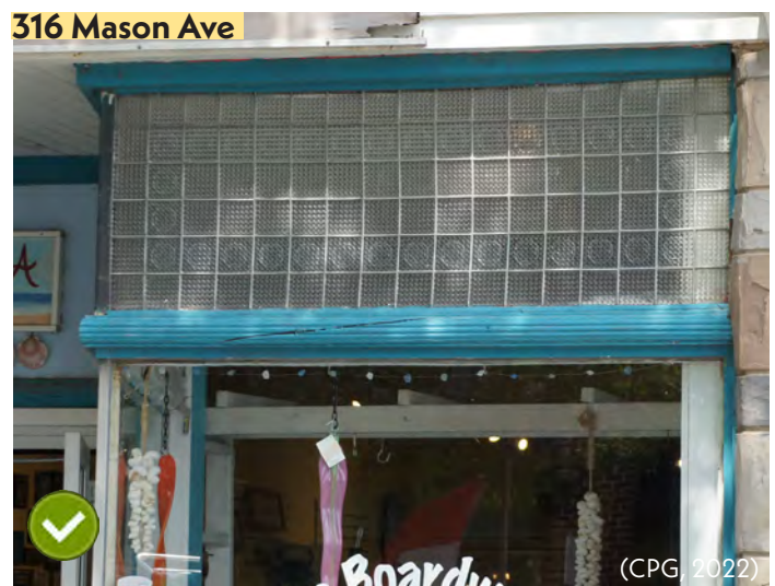
Figure 4.14 - Storefront transom windows, like the one shown above, are often painted over or covered by modern awnings that alter the historic storefront. These should be retained and repaired as necessary. If broken, a new glass pane should match the texture and size of the remaining historic panes.
