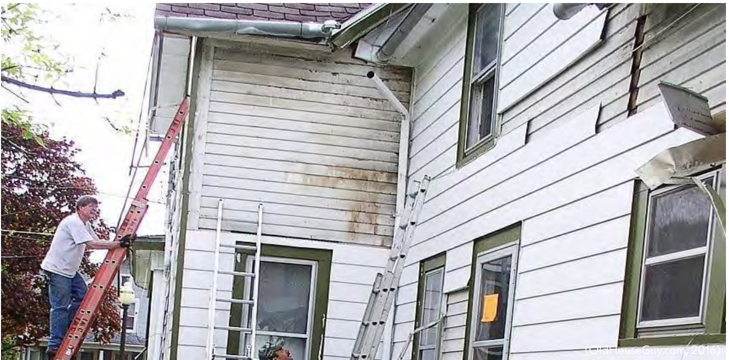
Figure 7.1 - Vinyl siding is not impervious to water infiltration. Above shows where lines of mold have stained the historic siding underneath the vinyl siding. Covering the historic siding has also changed the window and door profiles to appear flat. Alternative materials should be carefully reviewed and considered to avoid detrimental effects such as these.
