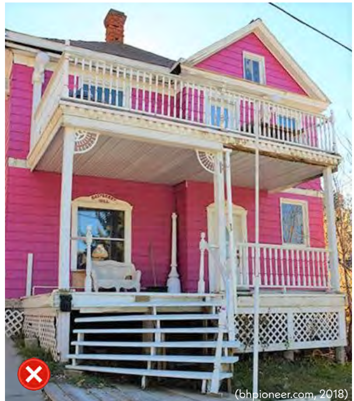
Figure 5.18 - Decorative ornamentation that is damaged or deteriorated should be replaced in-kind. Replacement materials of a different design change the appearance and character of a building, which is not appropriate.
