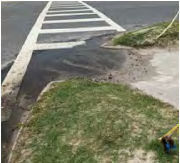
Storm water at a Mason Ave. crosswalk.
