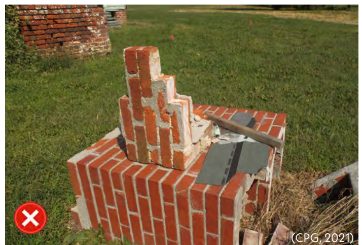
Figure 4.8 - Differing material strengths can often have a negative effect on existing materials. Here, a modern manufactured brick chimney top was added to a historic chimney and has since collapsed at the meeting joint of softer historic and harder modern material.
