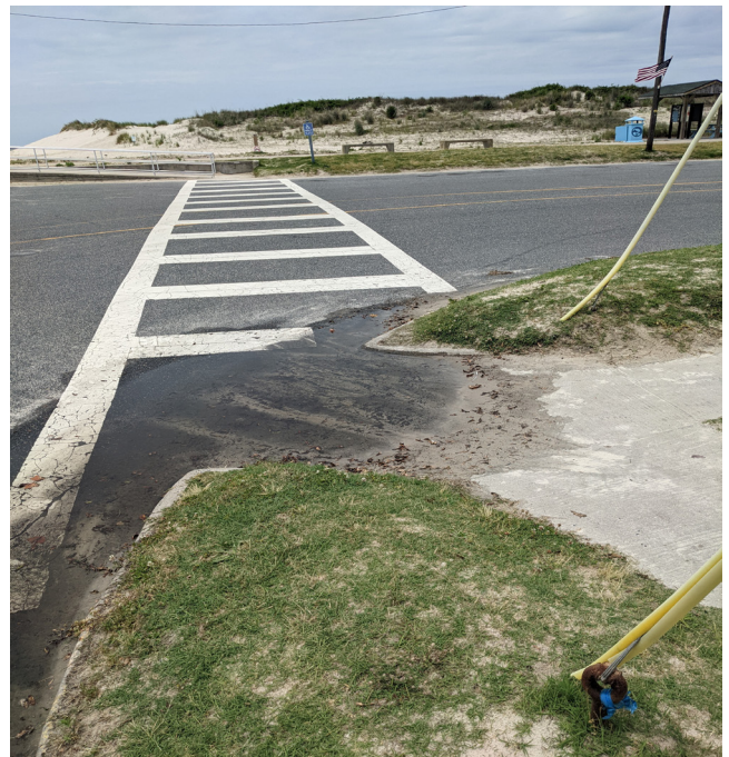
Storm water at a Bay Ave. crosswalk.
