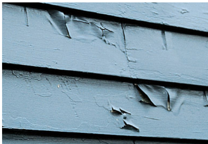
Figure 4.11 - The siding above has been painted when the wood was either too wet or there was a high level of humidity, resulting in bubbles and peeling of new paint.
