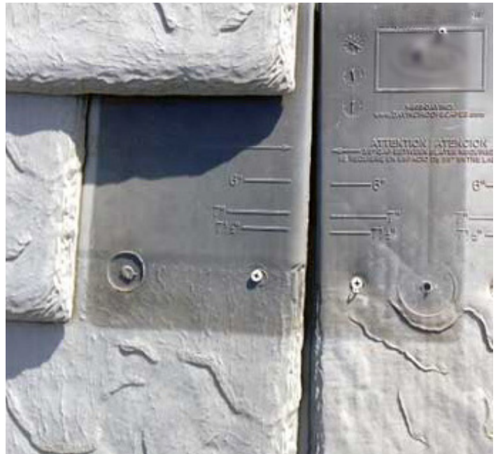
Figure 5.2 - Synthetic slate roofing is not an appropriate replacement material, as it has a tendency to warp (top photo), pucker, and bleach (bottom photo).
