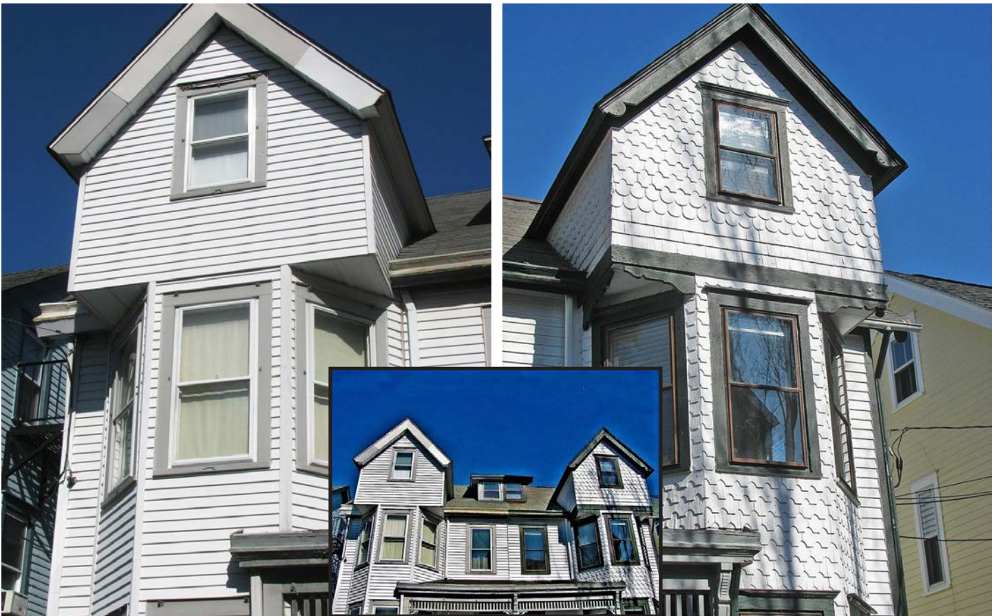
Figure 9.13 - The rowhouse on the right retains its historic wood shingles, decorative trim, and exposed rafter tails. The rowhouse on the left has been completely covered in vinyl siding. All ornamentation has been removed and the character defining features lost to the detriment of the individual resource and character of the overall Historic District. Alternative materials should be applied thoughtfully and only when necessary.
