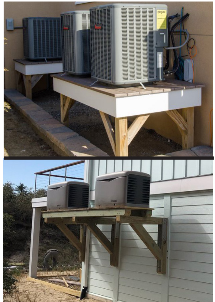
Figure 10.10 - Exterior mechanical equipment that needs to be raised should be located out of view from the public right of way and freestanding (top photo). Attaching brackets to a historic building is not recommended as it can strain and damage the structure.
