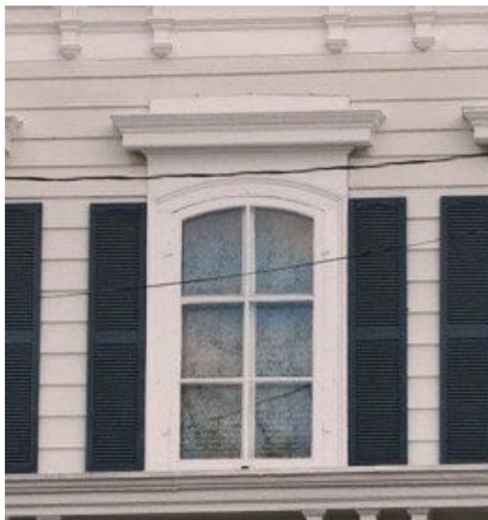
Figure 5.24 - An example of fixed shutters that are inappropriate for a historic resource. They are flat, mounted outside of the frame, do not match the shape of the window, and would not cover the width of the window if closed.
