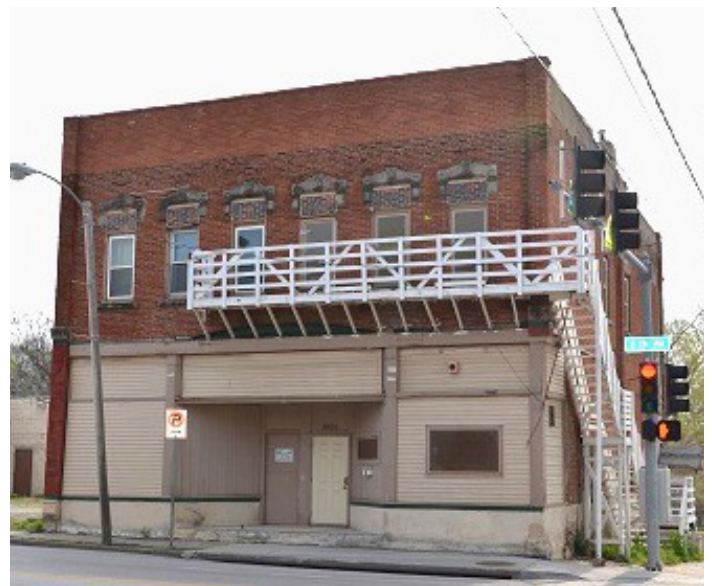
Figure 5.28 - This is an example of an inappropriate storefront modification. The display windows have been covered with modern siding, and the exterior stairs and balcony are an inappropriate alteration.
