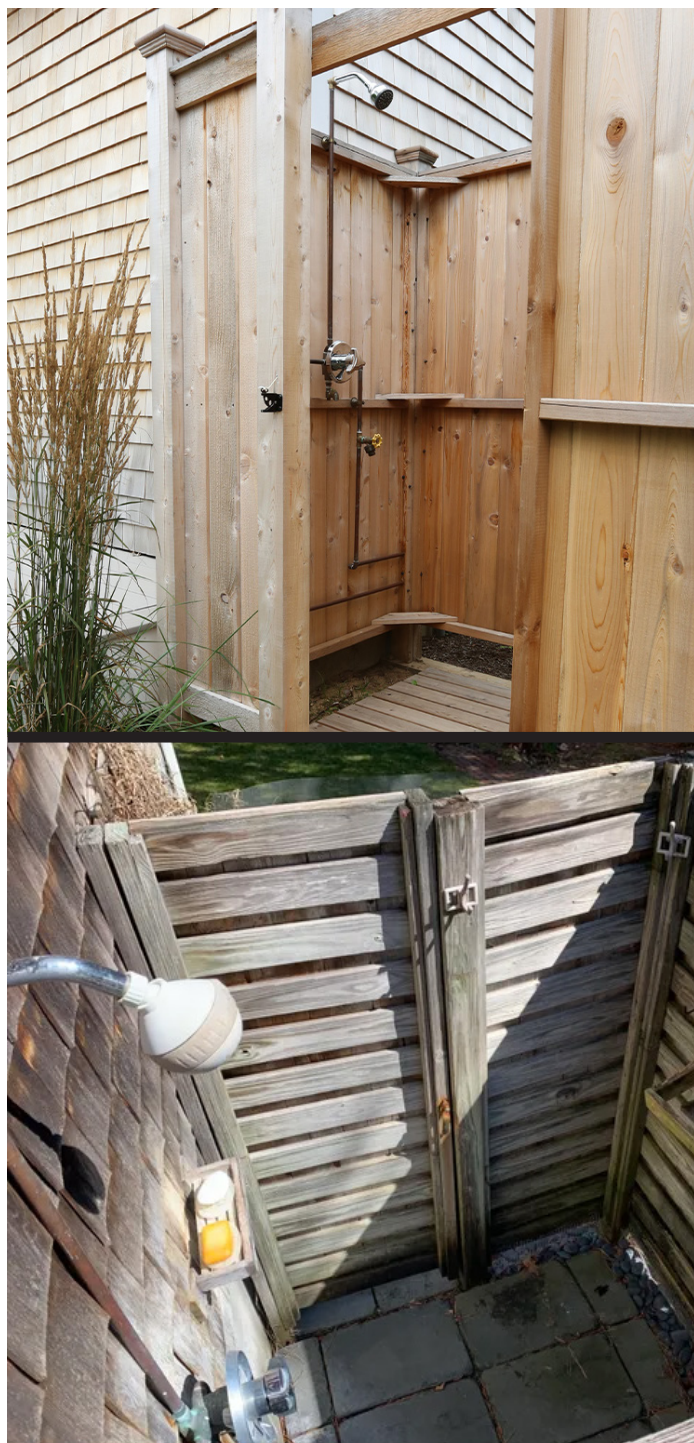
Figure 8.11 - The top outdoor shower has a built-out wood wall between the water and the historic shakes to protect from added moisture. The shower at the bottom has no protection and the shakes are visibly damaged from the added water and wear against them.
