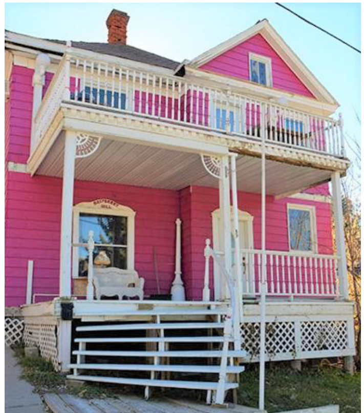
Figure 5.18 - Decorative ornamentation that is damaged or deteriorated should be replaced in-kind. Replacement materials of a different design change the appearance and character of a building, which is not appropriate.
