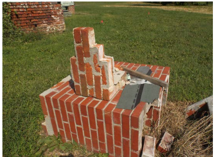
Figure 4.8 - Differing material strengths can often have a negative effect on existing materials. Here, a modern manufactured brick chimney top was added to a historic chimney and has since collapsed at the meeting joint of softer historic and harder modern material.
