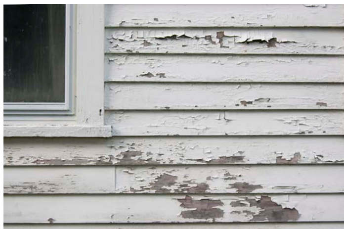
Figure 4.10 - This siding has weathered and peeling paint. It should be sanded down and repainted as soon as its deteriorating condition is noted so that the wood is not exposed to the elements.
