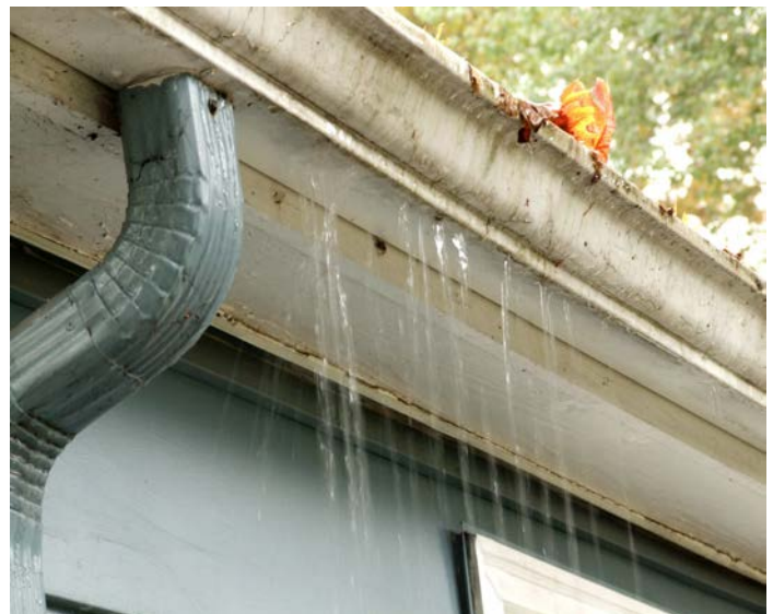
Figure 4.1 - The gutter shown above is clogged with leaves. These types of issues are easily fixed and will avoid excess water infiltration at the foundation.
