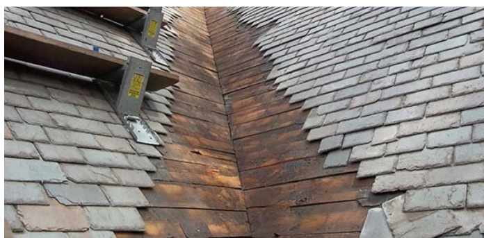
Figure 2.2 - Replacing a few broken or missing pieces of material, like slate tile (top), will save time and money by avoiding large costly projects such as a total-roof replacement (bottom), as well as foregoing the need to obtain a COA. Creating a regular maintenance inspection schedule will help detect these types of repair needs before it's too late.
