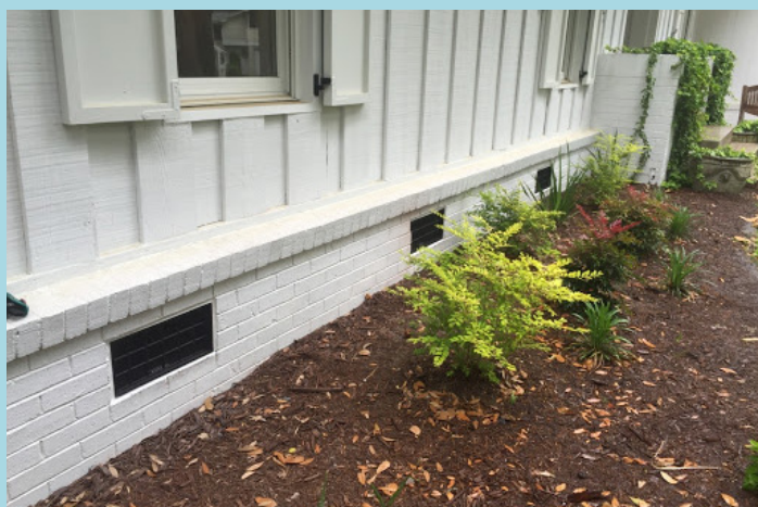
Figure 10.6 - Flood vents that allow water to move under the building is an example of wetproofing.
