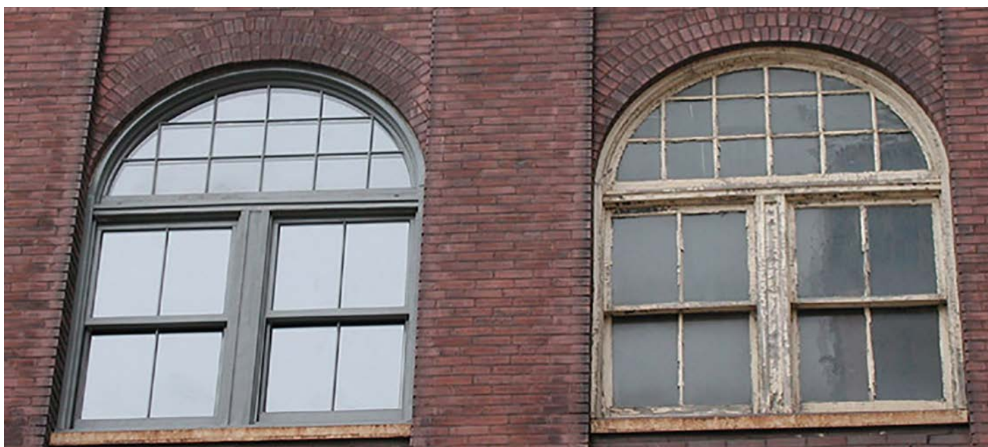
Figure 4.12 - The window at the left has been fully restored while the window at the right still needs work to be performed. Damaged and deteriorated windows can be salvaged.
