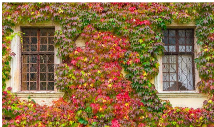
Figure 8.13 - Plants attached to historic materials can be detrimental to them. They hide possible deterioration and damage, impede repairs, trap moisture in their root system, and can weave into cracks making it difficult to remove. Using a trellis, frame, or wires installed near the building allows for the look, without the threat.
