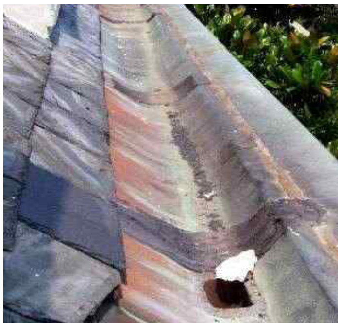
Figure 5.5 - An example of a built-in gutter in need of repair.
