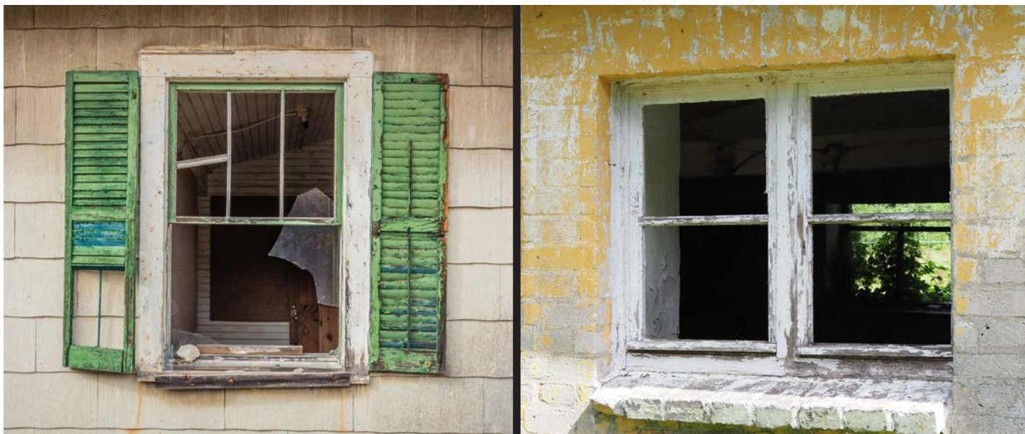
Figure 9.3 - If the windows above were on the same house, the one on the left would be approved for replacement as it is missing its lower sash, some of the upper sash muntins, all of the glass panes, and has significant sill damage. The window on the right, although missing panes and some paint deterioration, is still intact and salvageable. This one would need to be retained and repaired.
