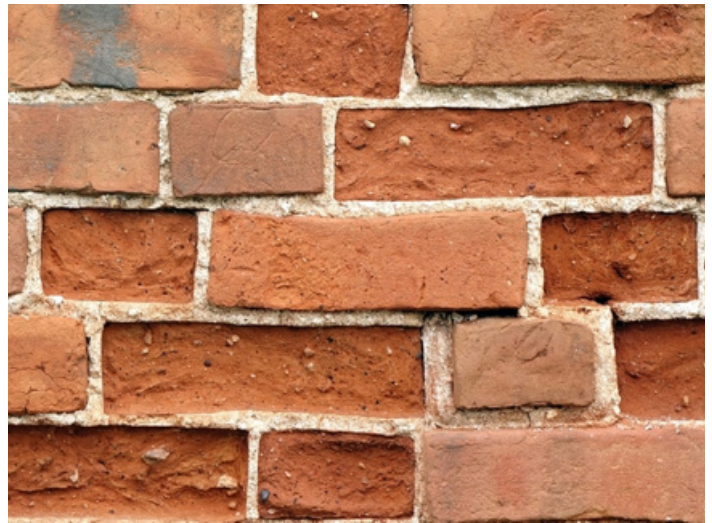
Figure 4.7 - Brick has surface layer, the brick face, that protects the softer, inside portion of the brick. When the brick face is damaged, which can occur when pressure washing at a high psi, spalling (shown above) occurs. The result is compromised bricks that flake and break away. When masonry requires cleaning, use a pressure of no more than 300 psi.
