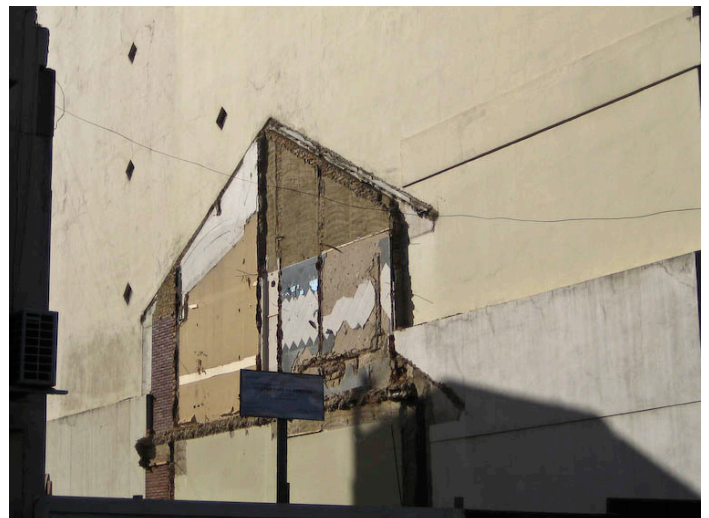
Figure 7.4 - Removing a building from the district creates a permanent hole in the historic fabric of the town. Too many these holes will eventually threaten the entire district's integrity that is irreparable.
